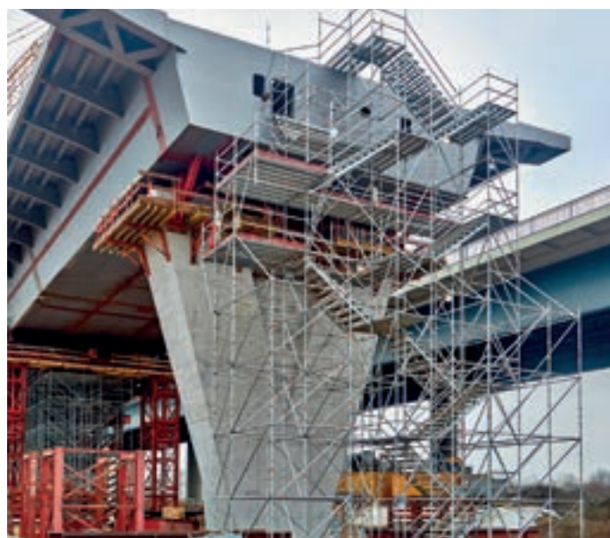
Site stairtower 200 for access to road surface, box girders and bridge bearings
