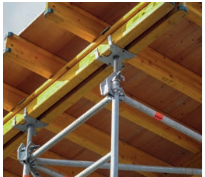
Shoring TG 60 as a slab table with pull-resistant connection of the formwork to the shoring towers
