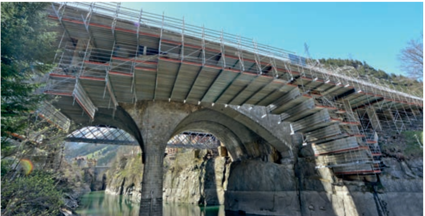
Bridge underside scaffolding with two levels made from Aluminium FlexBeam at a viaduct
