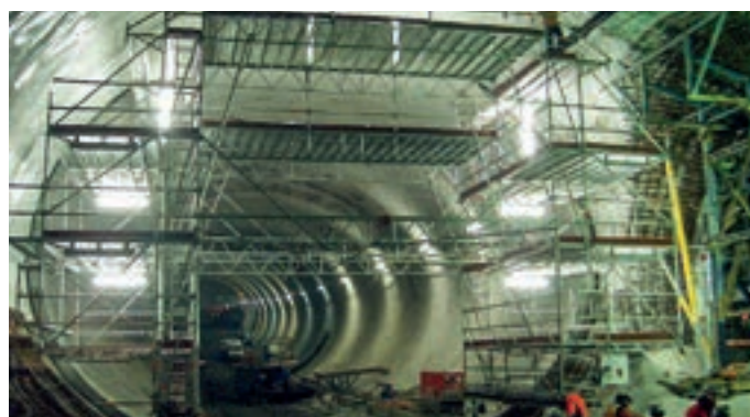
Mobile tunnel scaffolding running on rails with work platforms for safer working
