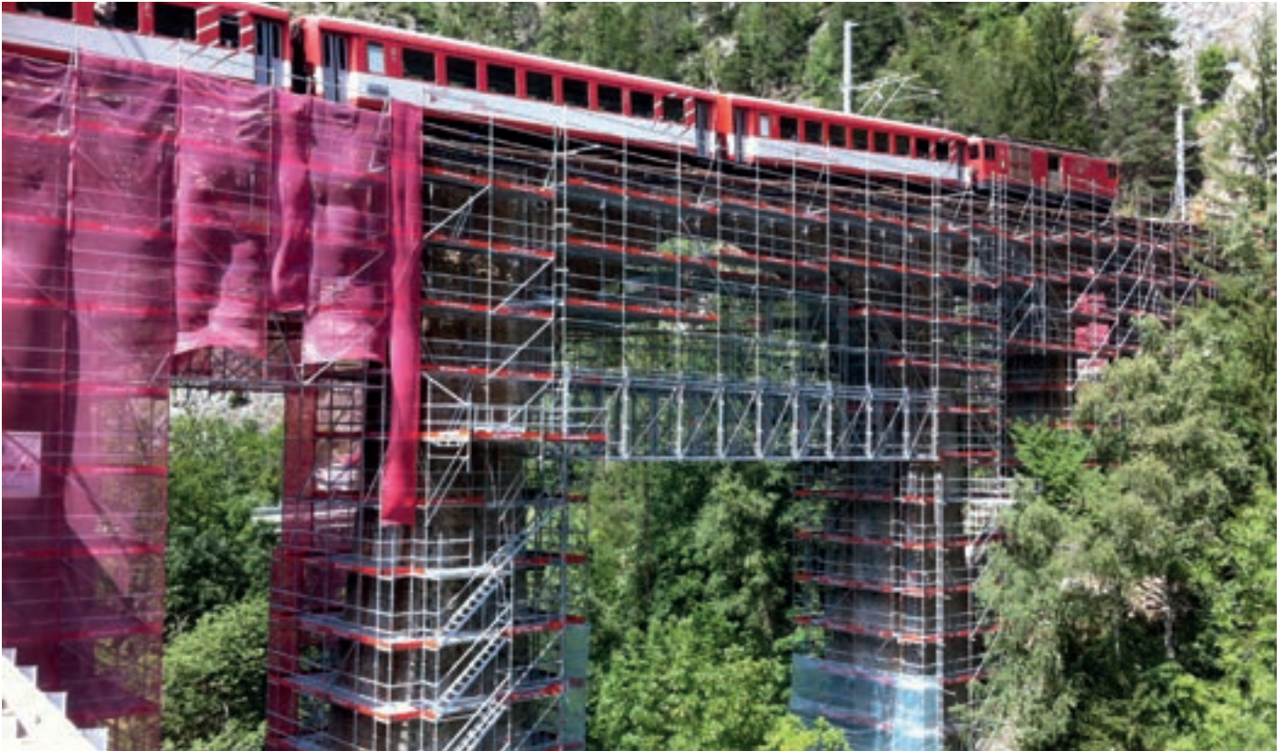
Free-standing work scaffolding on a stone arched bridge with Allround Bridging System for support
