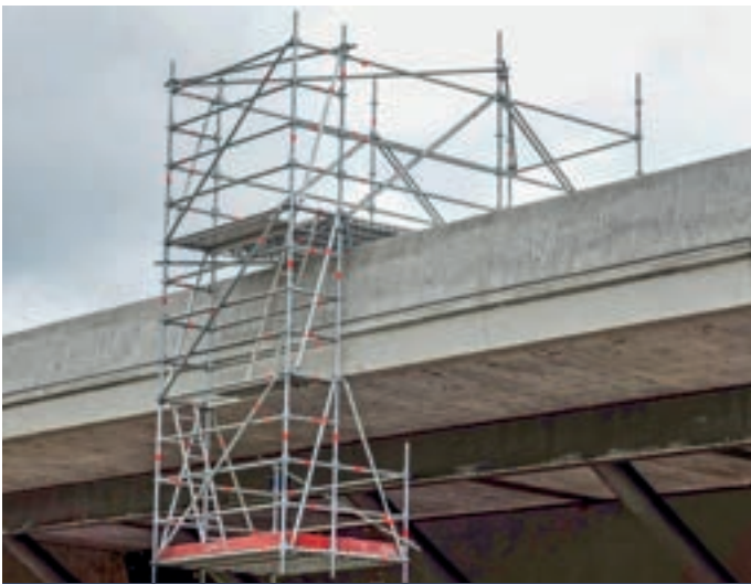
Mobile bridge cap scaffolding
