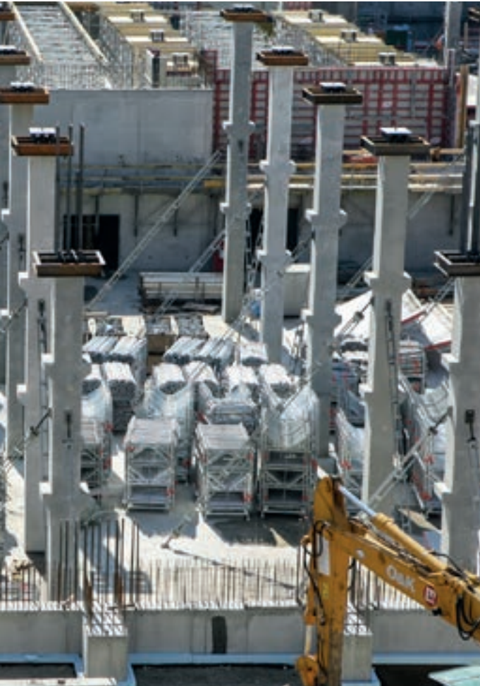
Filled pallets are lifted from the truck directly by a crane at the place of use.
