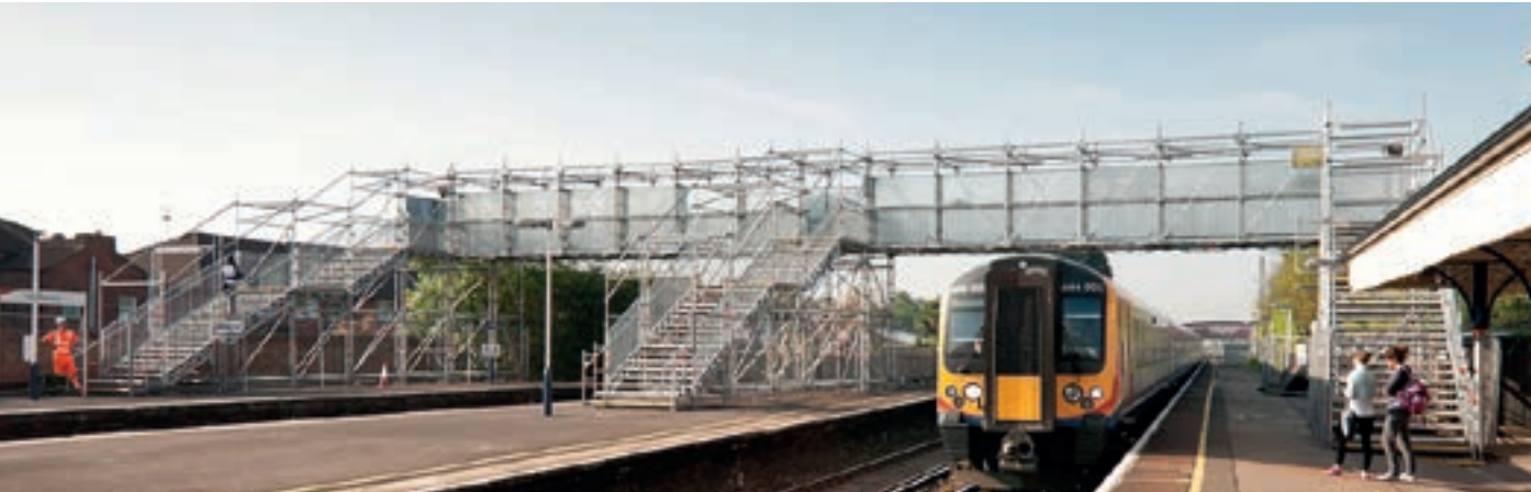
Temporary footbridge using Allround Bridging System on railway platform with Stairtowers 750 and internal Protect enclosure
