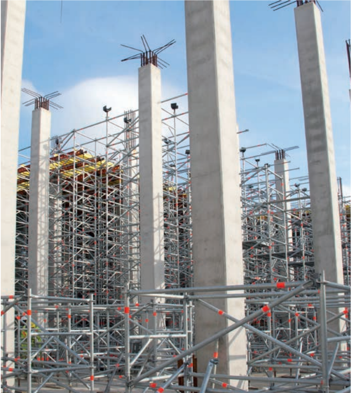
Connected shoring towers TG 60 during construction of a sewage plant – concrete pillars can simply be integrated into the shoring.
