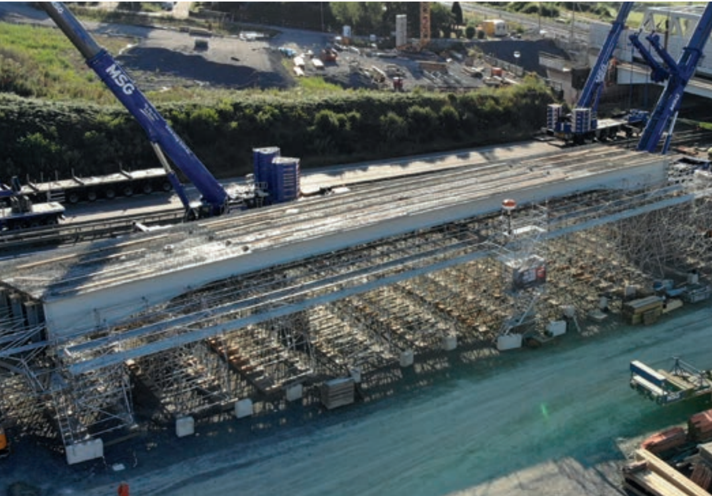
Shoring made from standard Allround components during construction of a new motorway bridge
