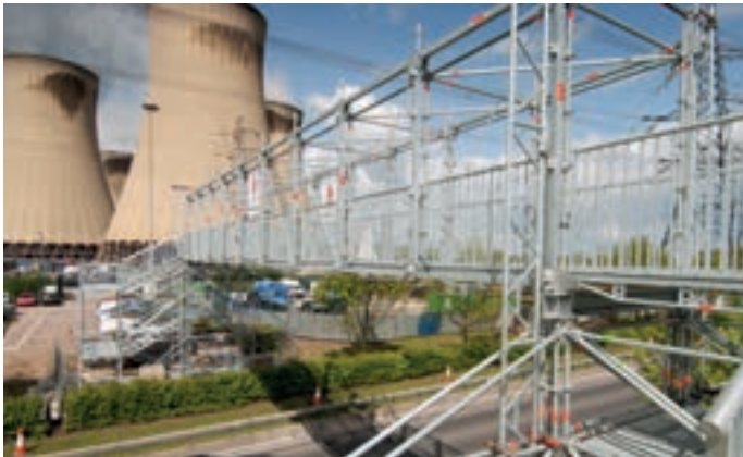
Temporary footbridge using Allround Bridging System with Stairtower 750 to assist site logistics
