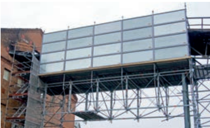
Work scaffolding covered using the Protect System on a pipeline bridge for fire damage repair
