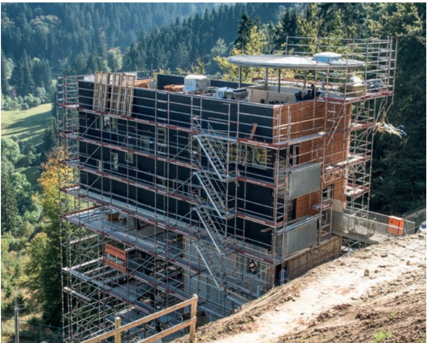
Allround work scaffolding in a complex terrain geometry, with integrated stair access
