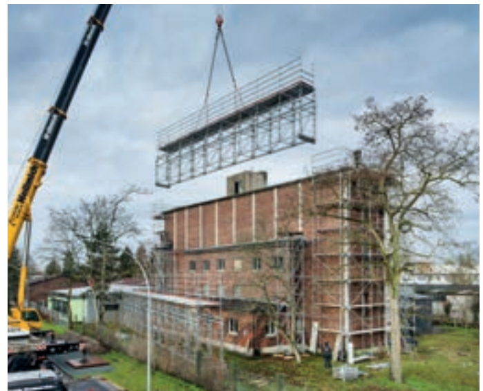
Bridging / supporting of work scaffolding using an external and non-loadable roof
