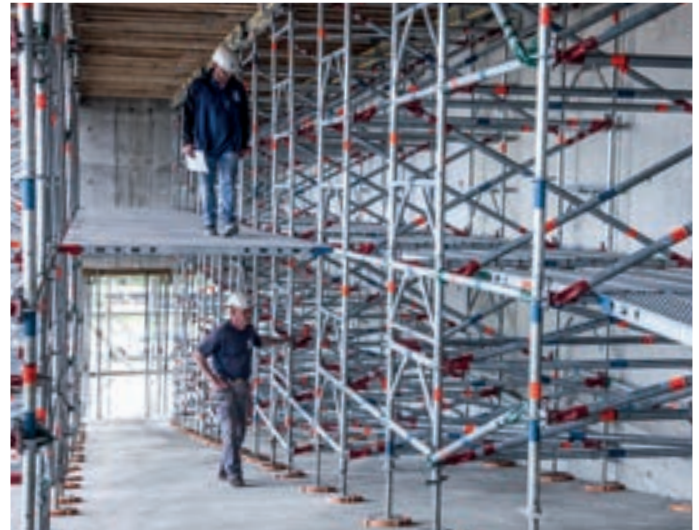
Integrated deck levels inside the shoring, and shoring adapted to the slope of the ground using equalising plates
