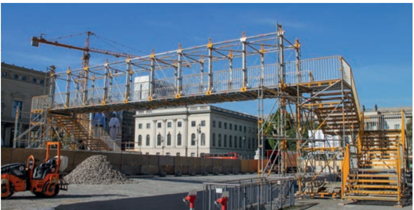
Temporary bridge over site with approx. 18 metre span to assist site logistics
