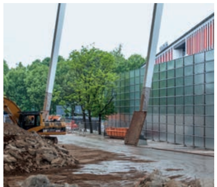
Noise and dust protection wall using Protect System, Mercedes Benz Arena, Stuttgart
