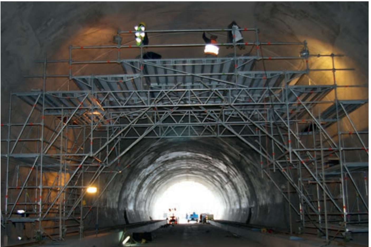
Mobile work scaffolding adapted to the tunnel geometry, with vehicle passage opening
