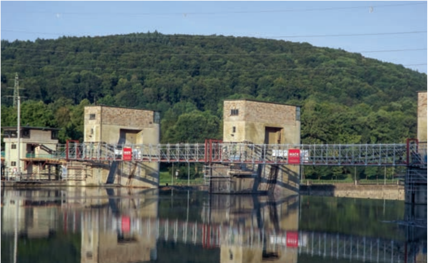
Temporary footbridge with a 2x 34 metre span and an intermediate section with Allround Bridging System
