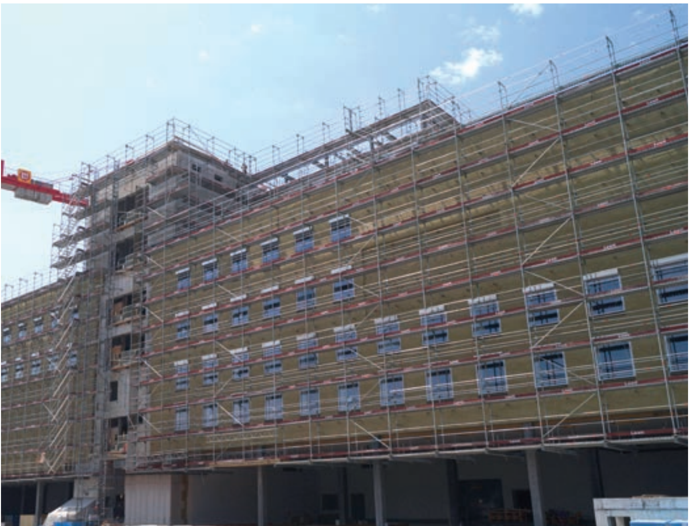
Facade work scaffolding of Layher SpeedyScaf resting on a projecting beam system to ensure continued vehicle access
