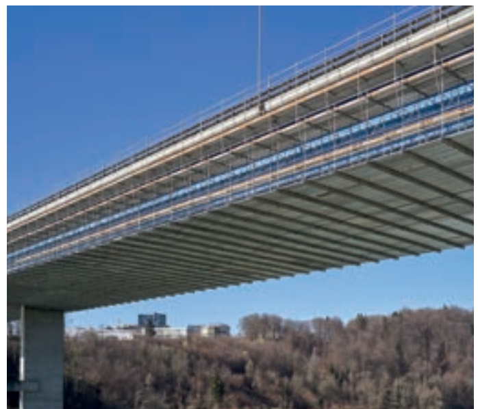
Approx. 7000 m 2 -sized bridge underside scaffolding with FlexBeam at a steel composite bridge
