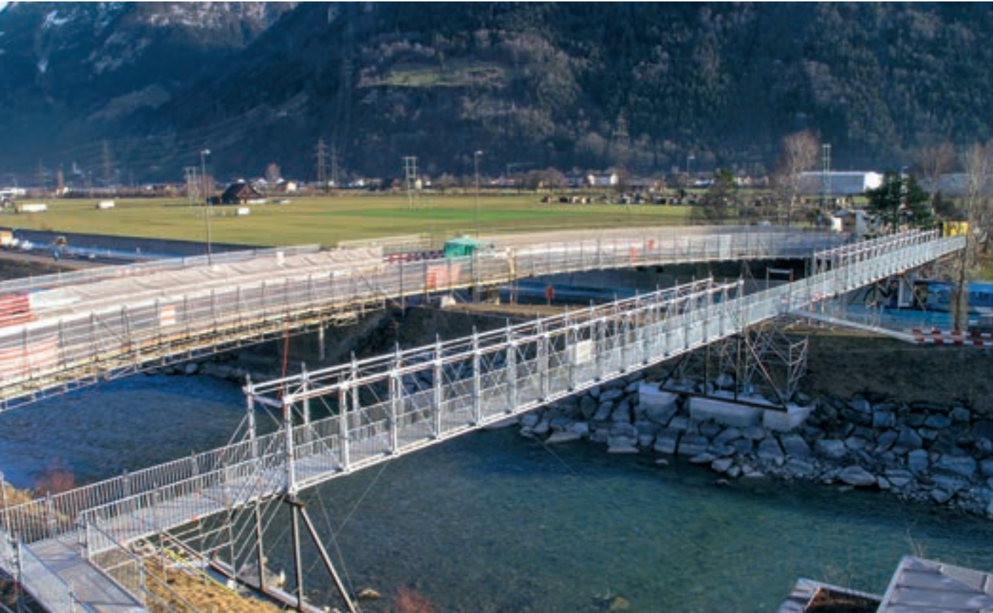
Temporary footbridge using Allround Bridging System with a span of 2 x 31 metres
