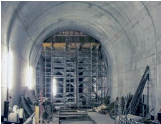
Pumped storage power station in Limmern, Switzerland
